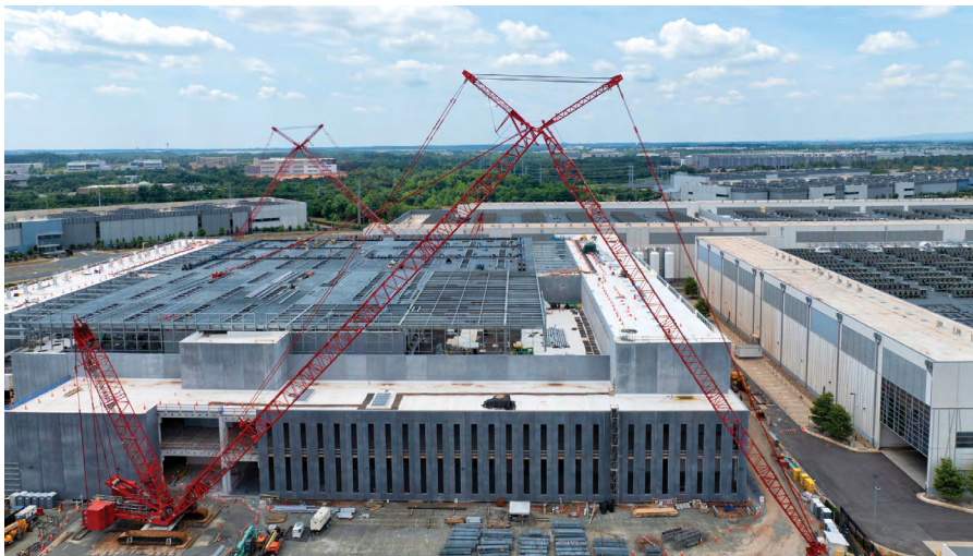
An aerial view of a data center being constructed inside “Data Center Alley” in the community of Ashburn, Virginia, located in Loudoun County.
