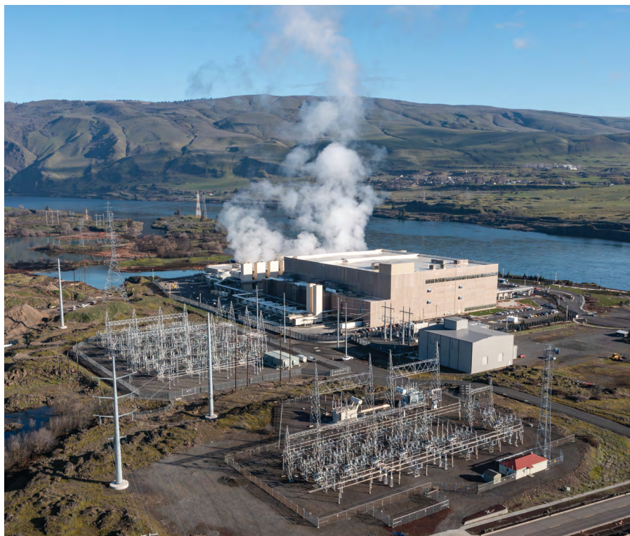
Data centers like Google's facility in the city of The Dalles, Oregon, depend on substantial energy, water, and physical infrastructure. Such demands are expected to grow as AI computing expands.
