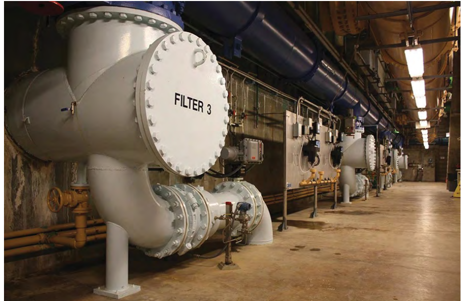
EXHIBIT 2 | Filter system at GWD's Corona Del Mar treatment facility 8
